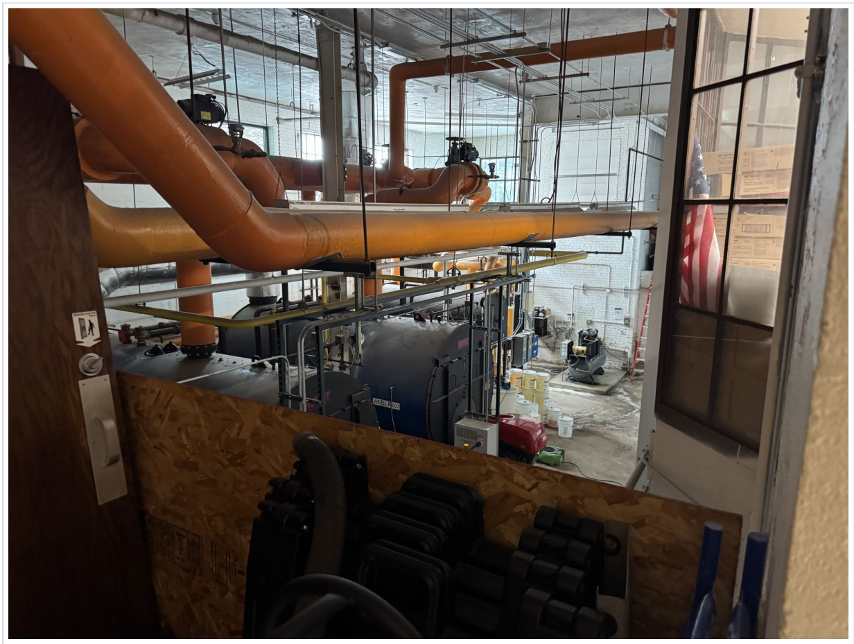
Figure 3.1 — Figure 1: weeping compression joint below the low-loss header
