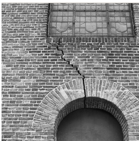
North elevation showing the stepped crack at grid C
