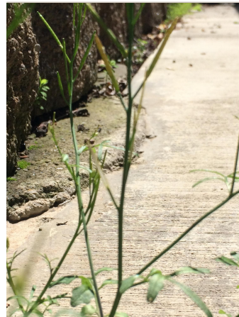
Crack C1 with tell-tale installed
