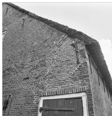
Crack C1 with tell-tale installed
