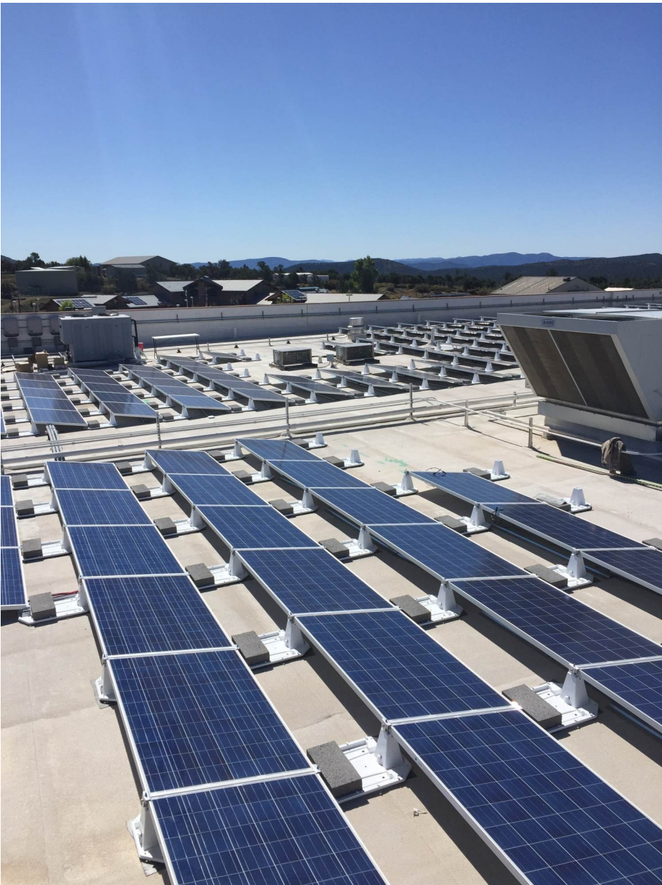
Figure 4.1 — Bird soiling on module 1-7 at the time of inspection
