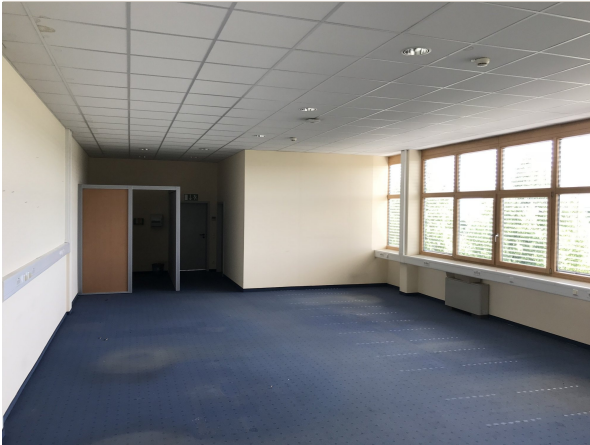
Stained ceiling tiles below the AC cassette
