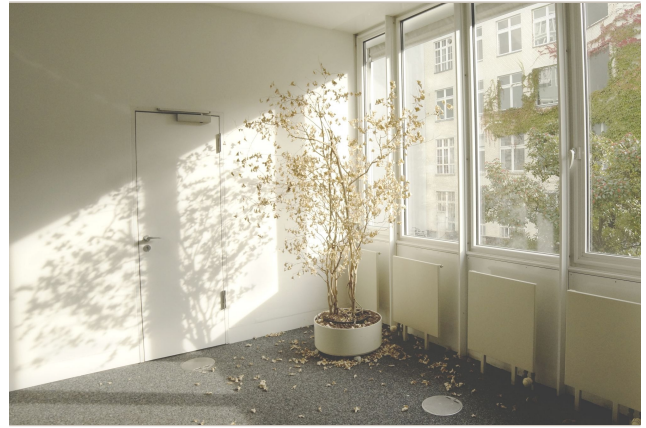
Holes left by removed fixings
