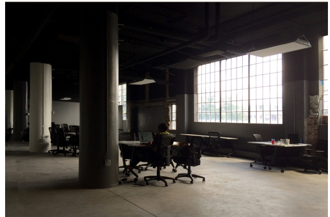
Holes left by removed fixings
