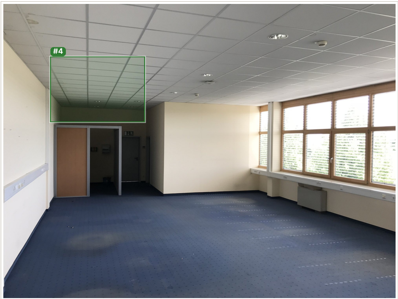
Photograph 3 — Stained ceiling below the AC cassette (appendix)
