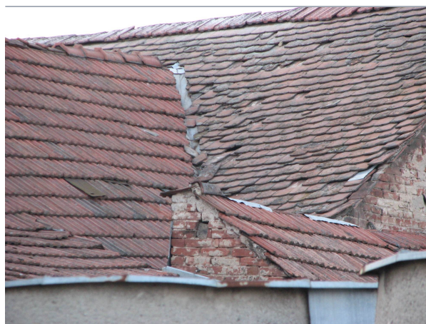
Slipped tiles to the rear slope
